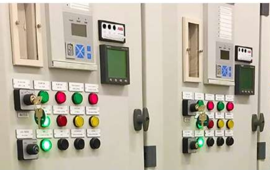
Control Panel Manufacturer
